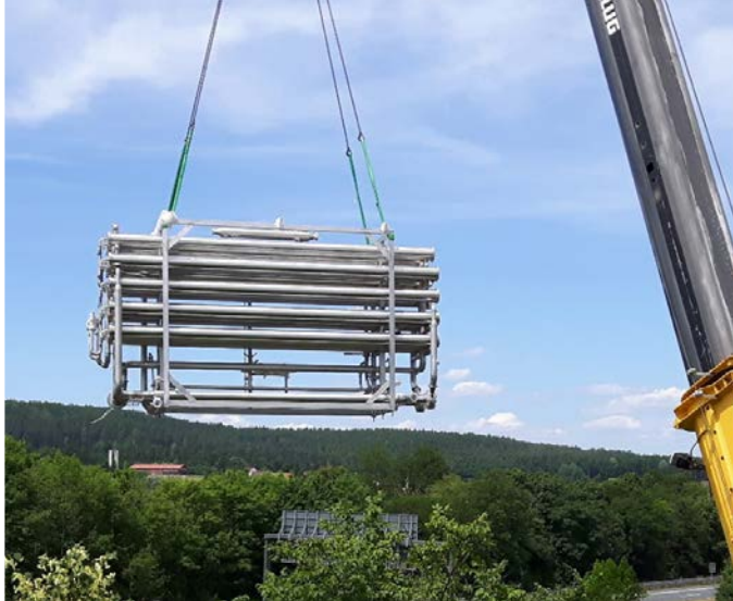
Installation of the second RO High TS -plant for the concentration of whey
